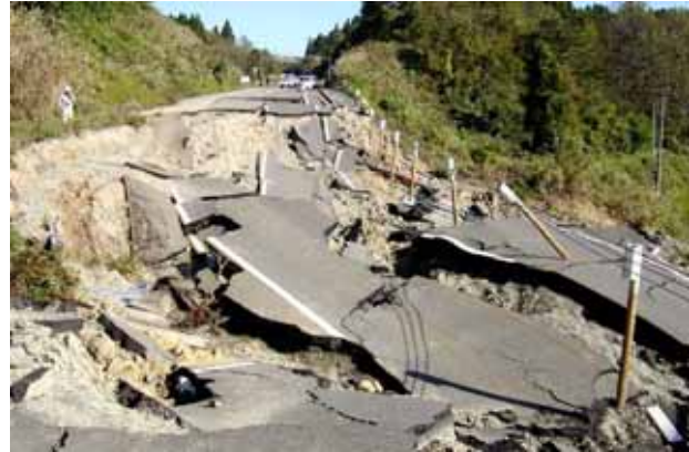
Blocked route by the 2004 Mid Niigata Prefecture Earthquake
