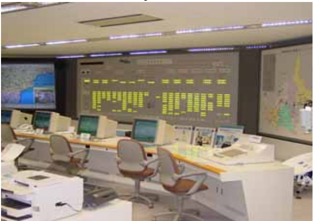
Communication Control Room
