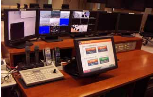
Shizuoka Pref. Crisis Management Center (East) AV operation desk
