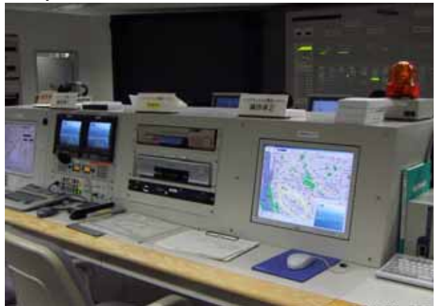
Helicopter TV Transmission System established by prefectural government control bureau (communication control room)
